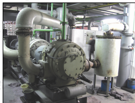
Old Wittig pump, replaced by UV50 in 2004
