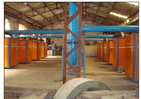
Pumps Room with 10 x UV50 VS90 HC
