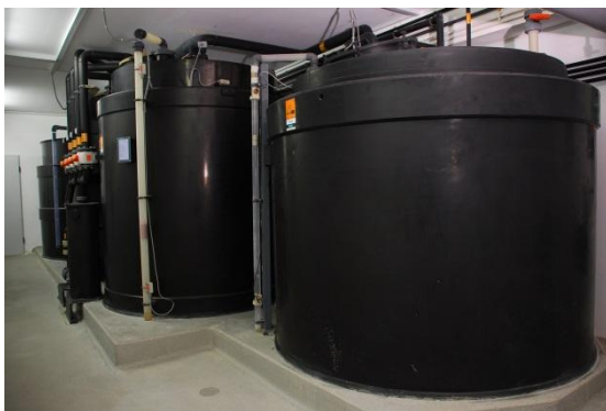
Fig. 3: Neutra chemical storage tanks
